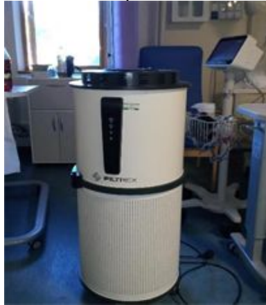
Air Scrubber in place at St Richards Hospital
